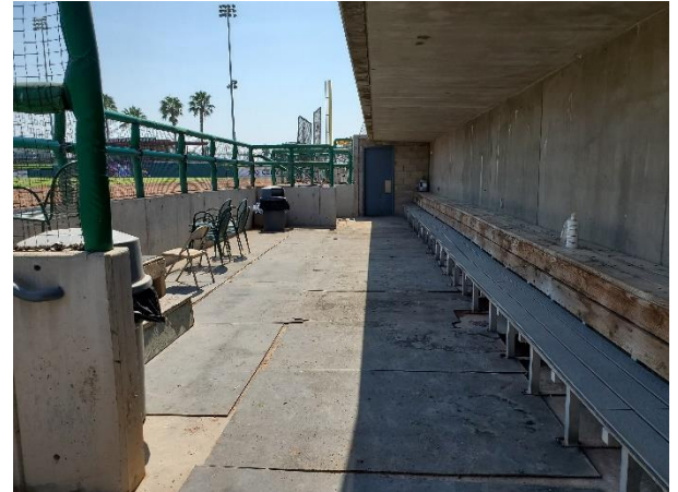
SECTION 7.5: THE DUGOUT HAS ANTI-SKID FLOORING BUT THE RUBBER MATS ARE LOOSE WITH GAPS AND PRESENT A TRIPPING HAZARD.
