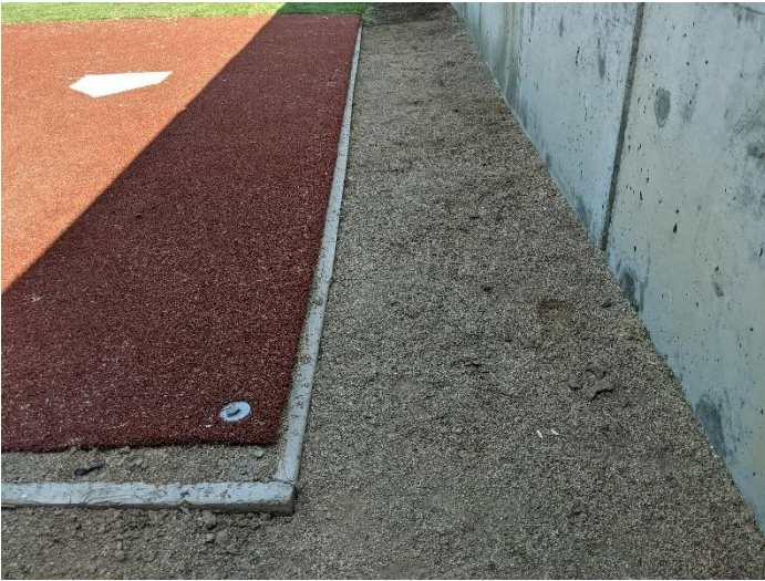
SECTION 7 (PLAYING FIELD) – ADD ADDITIONAL MATERIAL AROUND WOOD CURB in BULLPEN– TRIPPING HAZARD
