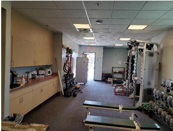
SECTION 3.2: HOME COMMISSARY AND DINING AREA IS NOT SEPARATED FROM THE LOCKER RM (IS IN THE WEIGHT RM) IS MISSING MUCH OF THE REQ'D EQUIPMENT AND HAS NO SEATING.
